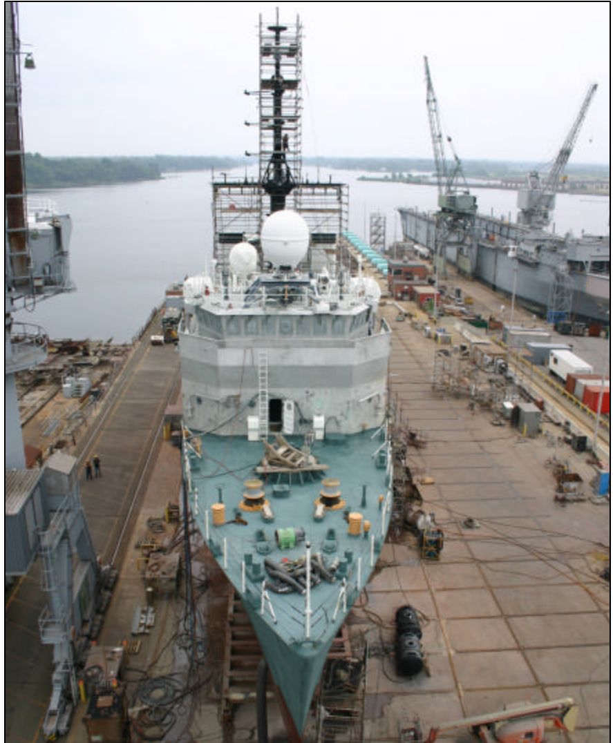
The medium endurance cutter USCGC Tampa (WMEC 902) sits high and dry at the Coast Guard Yard in Baltimore, Md., during a nine-month major systems refurbishment as part of the Mission Effectiveness Project (MEP) for 210-foot and 270-foot medium endurance cutters. In addition to the cutter’s refurbishment, the Coast Guard’s Engineering Logistics Center is conducting a concurrent Integrated Logistics Overhaul. (Photo by Gordon I. Peterson)
